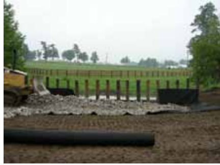
Figure 7. The posts are reinforced with geotextile fabric and rocks, which form a base for the soil.
