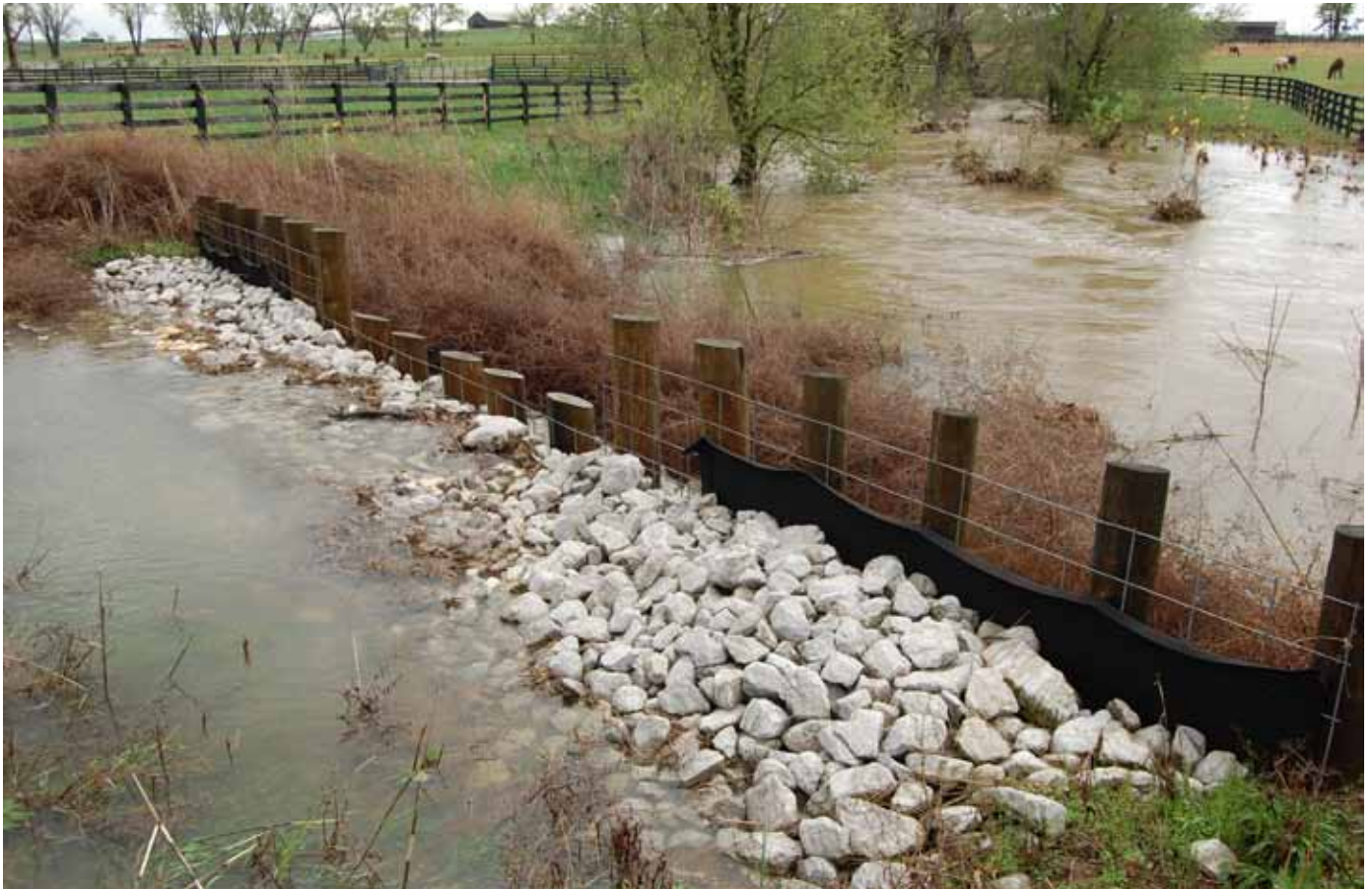
Figure 9. The completed grade stabilization structure prevents erosion by controlling the flow of water, absorbing stream energy, and controlling the elevation change.
