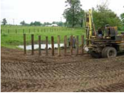
Figure 6. Posts are installed to support the bank in a grade stabilization structure.
