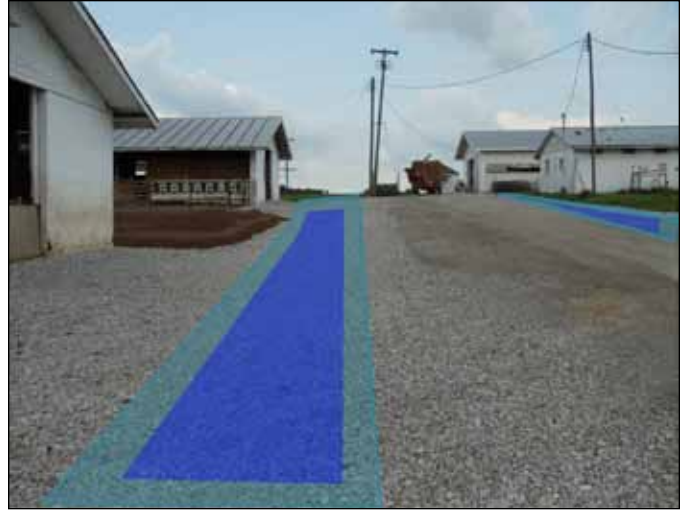
Figure 2. This rock-lined channel diverts clean water away from the production area (left) and prevents erosion near the buildings.
