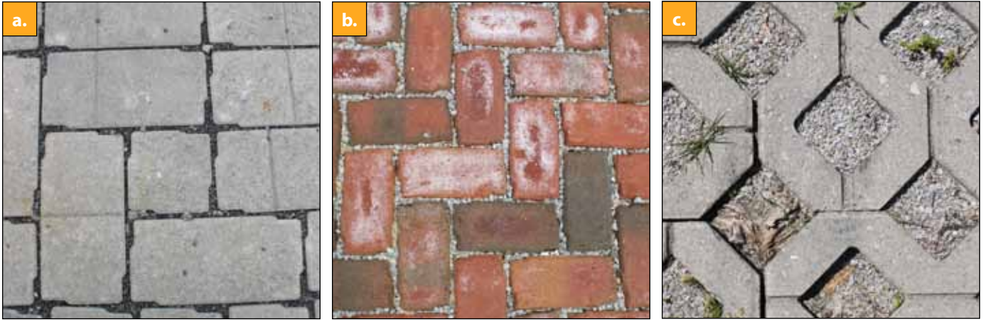
Figure 6. (a) Permeable interlocking concrete pavers (PICP), (b) permeable interlocking clay brick pavers (PICBP), and (c) concrete grid pavers (CGP).
