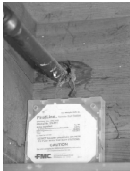
Fig. 5. Typical aboveground placement of a FirstLine Termite Bait Station.
