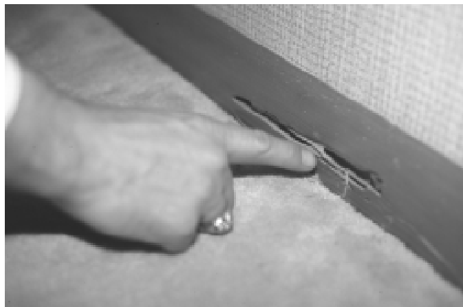
Fig. 2. Termite damage to baseboard, discovered by the homeowner while vacuuming.
