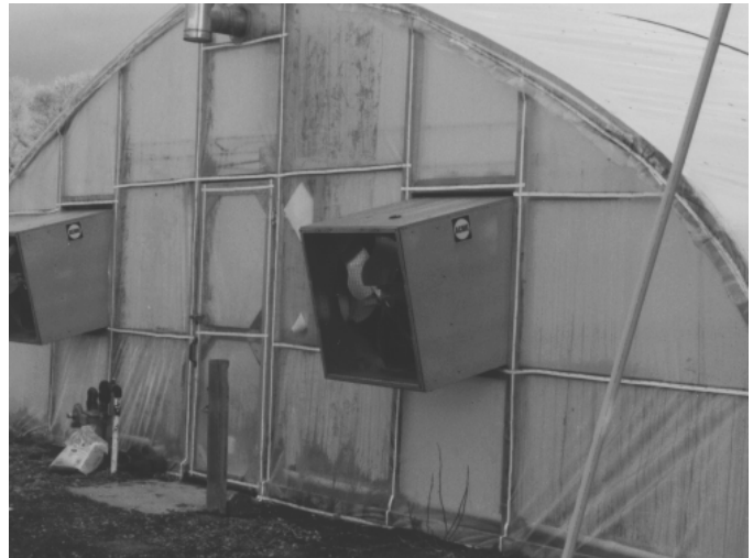
Figure 14. Vent fans in end wall.
