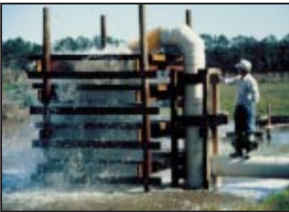
Figure 3. Aeration screens used on pump discharges.
